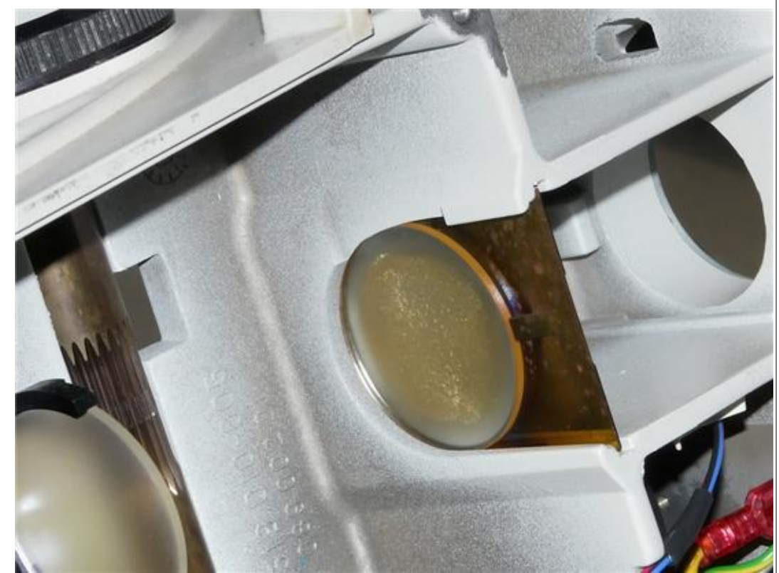
(3) Inspect the diffuser in the center of the photo above. The one shown has severe heat damage, being cracked and yellowed.
