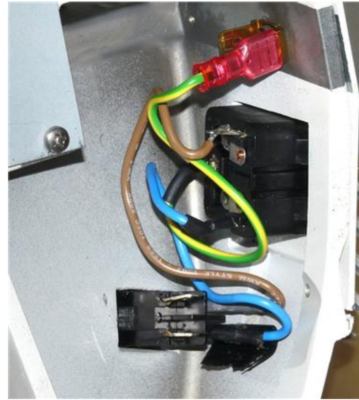
(2) Remove all of the AC Power connections from the AC receptacle shown in the picture above. The power connections to the power supply have already been removed by unplugging the power cable.
